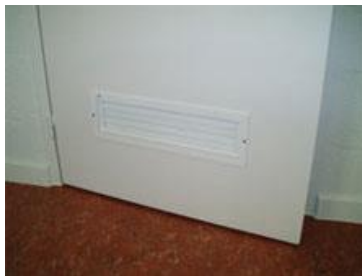
Doorstroomopening in deur
