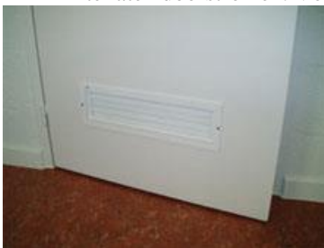
Doorstroomopening in deur
